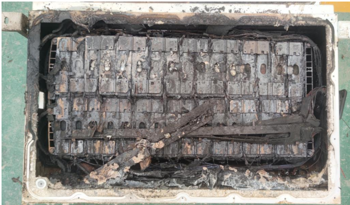
Internal view of initiating module, after test
